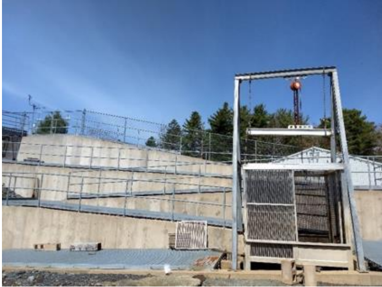
Figure 2. Left - Hebb Dam Fish Passage Trap lifted out of passage with the door open.
