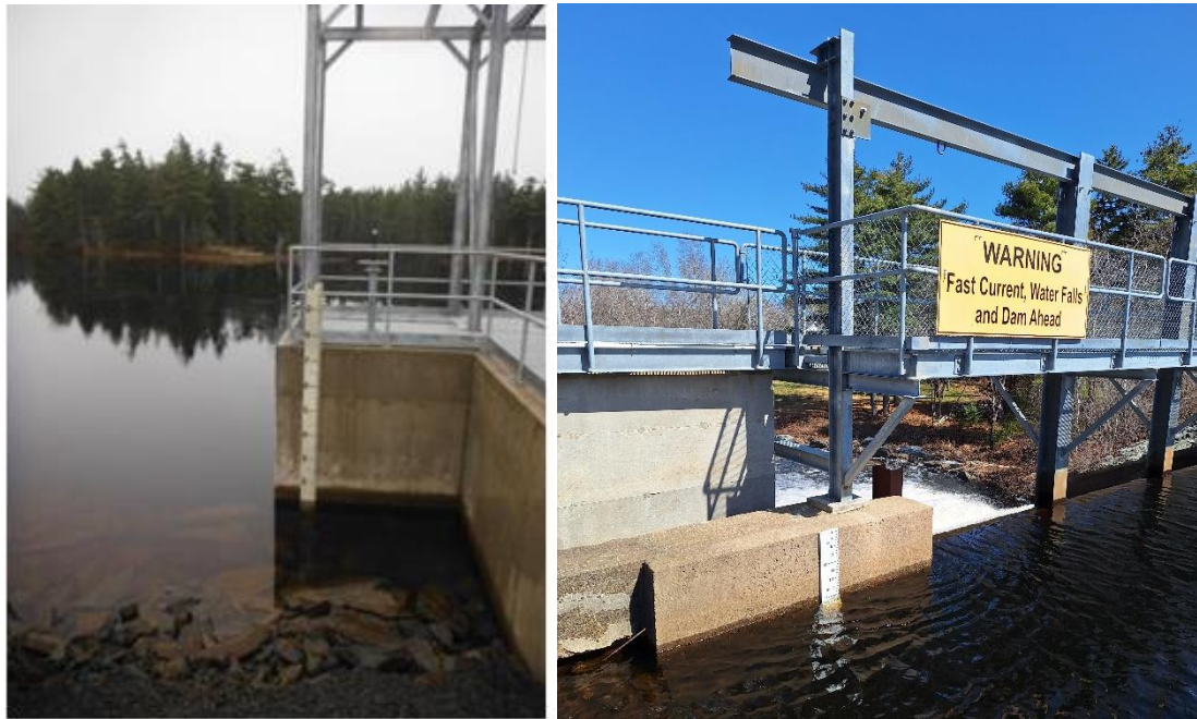
Figure 3. Previous (left) and new (right) water level gauges above Hebb Dam near fishway exit.
